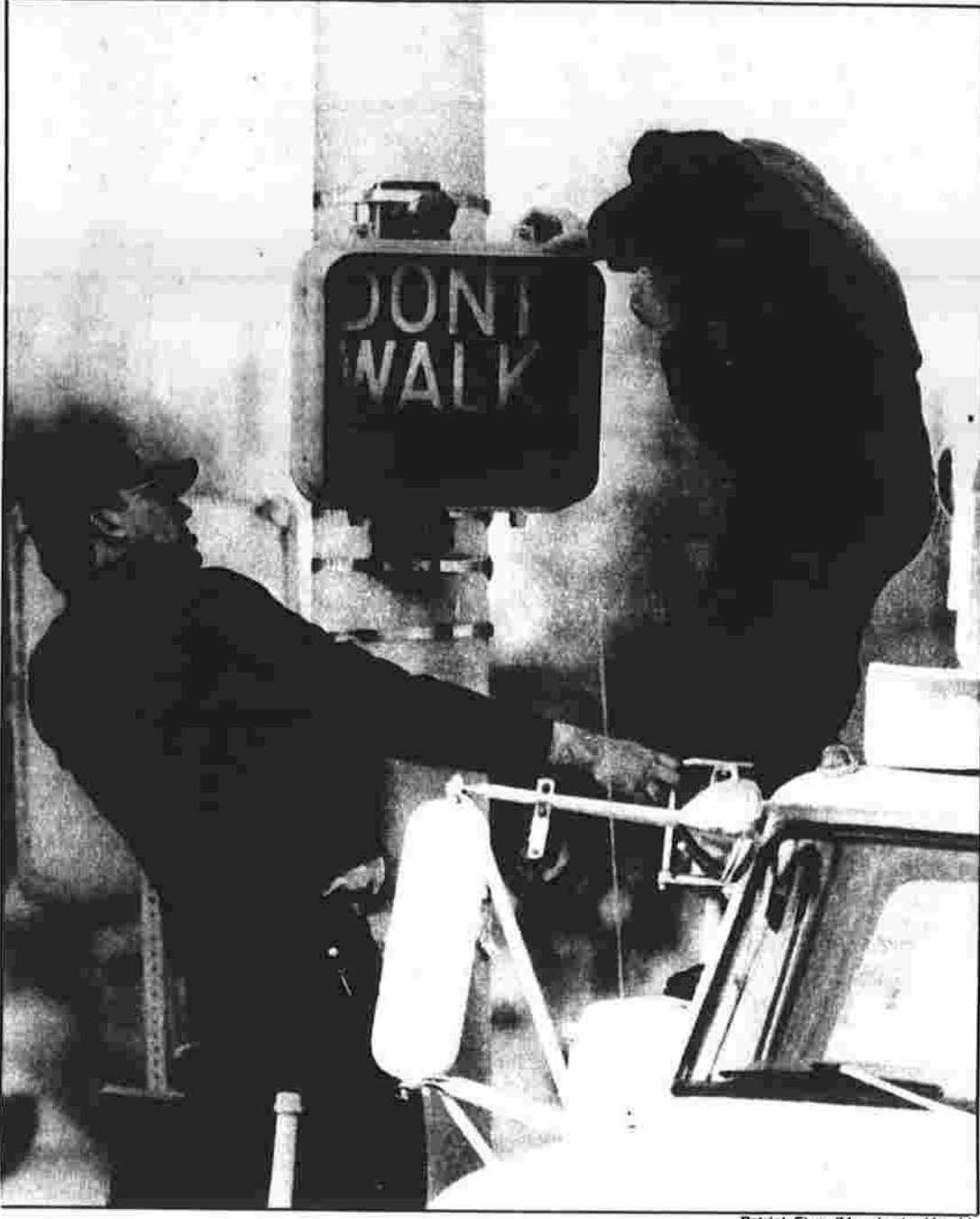
CROSSED SIGNALS — Dave Foreman of 299 E. Middle Turnpike and Bob Leger of 239 E. Middle Turnpike, employees of the Manchester Police Department, repair a crossing signal Friday at the intersection of Middle Turnpike and Main Street. The two said the signal was damaged recently when a trailer truck struck the pole.
